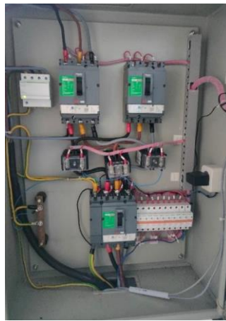
Gambar 9. Panel Kontrol Output Inverter.
